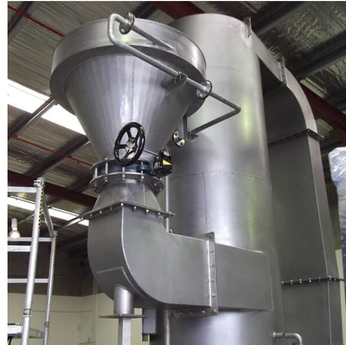
Figure 7. Venturi wet scrubber 33
